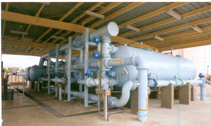
IRON AND MANGANESE REMOVAL SYSTEM EQUIPMENT CONSISTS OF THREE 84-INCH DIAMETER FILTER VESSELS WITH STAINLESS STEEL WEDGE FLOW LATERALS, ELECTRIC OPERATED VALVES, FLOW METERS, FLOW CONTROL VALVES, AND A PLC FILTER SYSTEM CONTROL PANEL FOR FULLY AUTOMATIC OPERATION.
