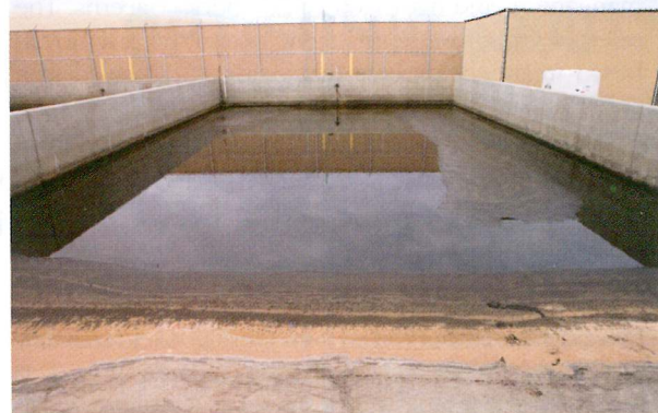
ONE OF THREE SOLAR DRYING BEDS USED FOR THE AGUA VIVA WATER TREATMENT FACILITY INTERIM PHASE IMPROVEMENTS. SLUDGE IS PUMPED FROM THE BACKWASH WATER RECLAIM SYSTEM INTO THE DRYING BED FOR DEWATERING BY SOLAR EVAPORATION. THE PROCESS HAS PROVEN SO EFFICIENT IN THE CITY OF YUMA THAT ONLY TWO OF THE DRYING BEDS ARE CURRENTLY USED.
