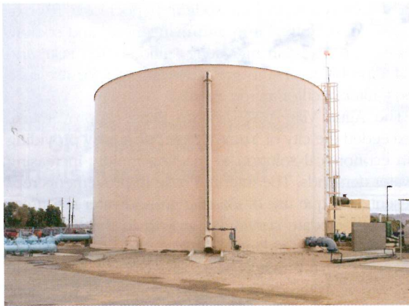
SPENT BACKWASH WATER IS PUMPED FROM THE FILTER VESSELS TO A RECLAIM STORAGE TANK. BACKWASH WATER IS GIVEN ADEQUATE TIME FOR SUSPENDED SLUDGE TO SETTLE TO THE BOTTOM OF THE STORAGE TANK. THE CLARIFIED WATER IS RECLAIMED AND PASSES BACK THROUGH THE FILTER. SLUDGE IS THEN PUMPED FROM THE STORAGE TANK TO SOLAR DRYING BEDS.
